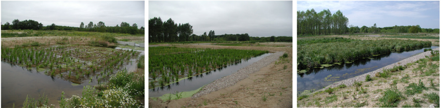
Installation and planting of the floating elements have been accomplished in 2005. Throughout the first year after installation the vegetation has matured forming a dense stand of plants.
