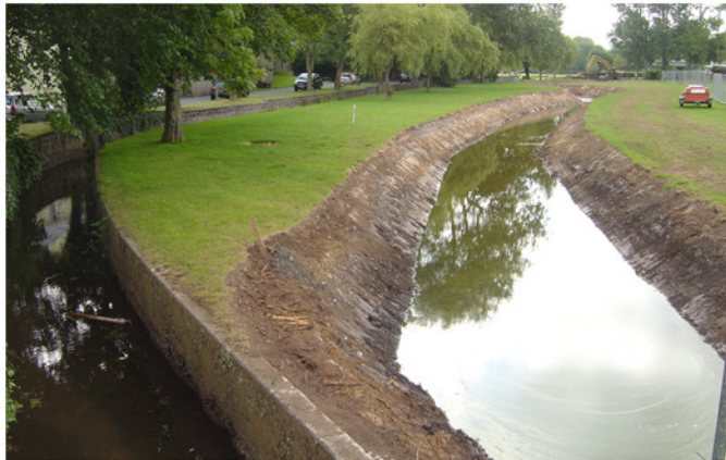
Above: The old concrete channel (left) and newly cut sinuous channel (right)
