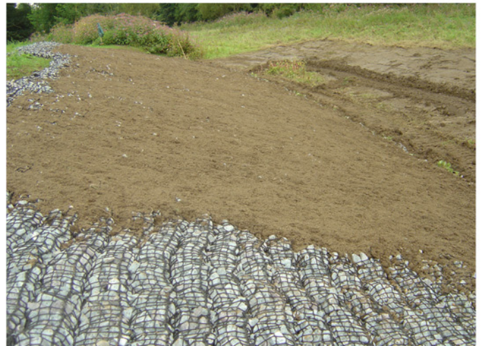
After the placing the mattresses are covered with topsoil and seeded to blend into the environment.
